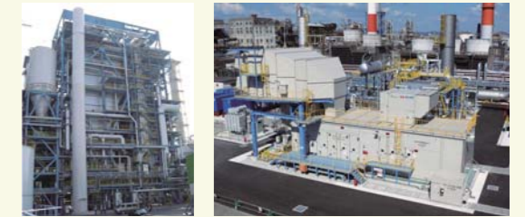
Circulation fluidized bed boiler at the Ohtake Plant
